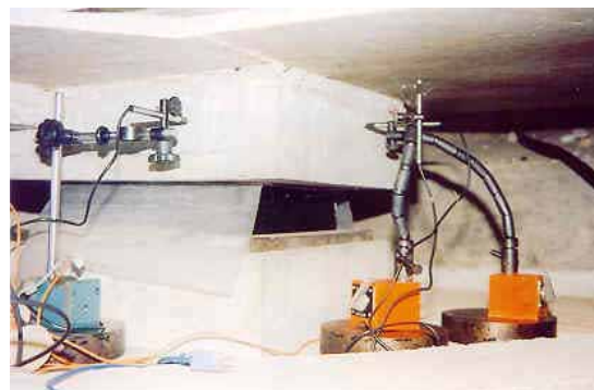
Figure 4: Sensors for measuring displacements on a bridge bearing.
