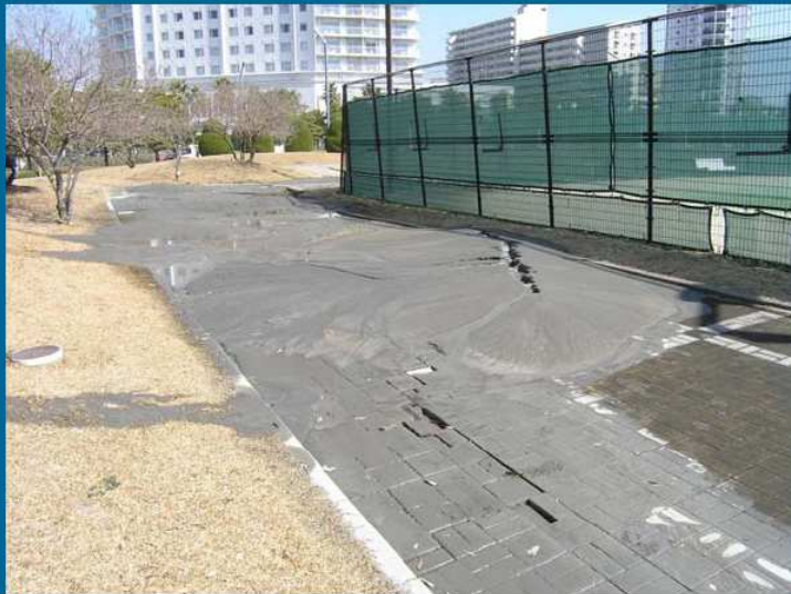
Liquefaction in young sandy deposit (Urayasu City near Tokyo)
