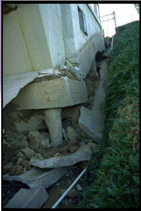
Karl V. Steinbrugge Collection, Earthquake Engineering Research Center
